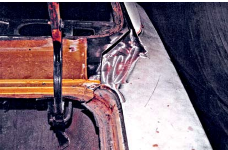
This is the right side of trunk drain; the tin worm had rotted out this piece; Watson, again, precisely cut, carefully welded and made metal fit like new
